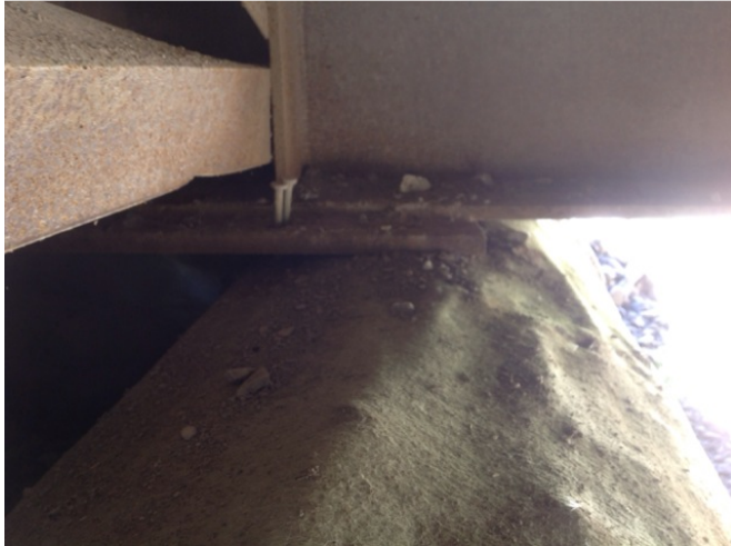
left downstream bearing
